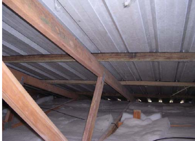
Figure A.6 Although the roof was ventilated by two wind driven ventilators at the eaves this was insufficient to prevent condensation.
