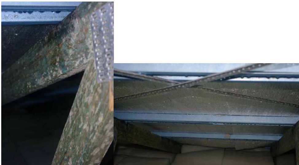
Figure A.8 Mould growth on roof trusses and condensation on the underside of the foil sarking
