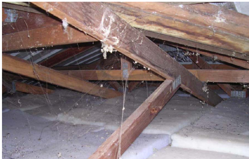
Figure A.5 Insulation in the south east corner of the roof space restricted eaves ventilation
