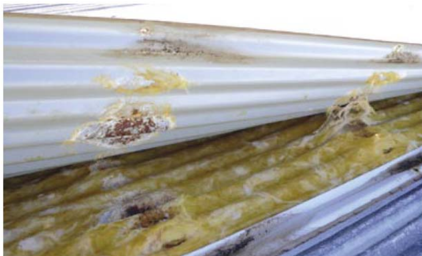
Figure 5.6 Photo showing moisture penetration due to the absence of a vapour barrier in a tropical environment
